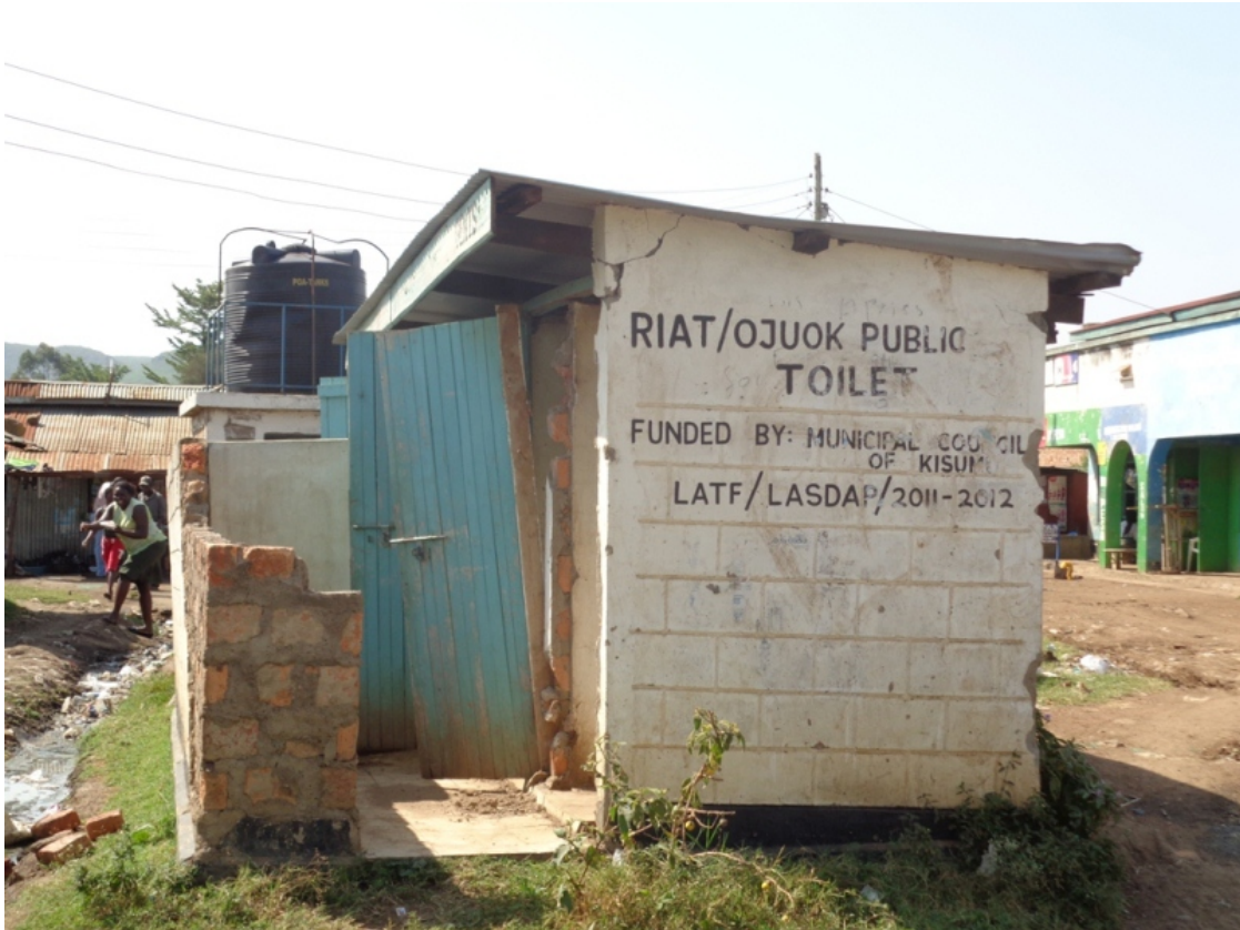
Plate 5: Dilapidated pit latrine in Ojuok Slums near Kisumu Airport. In the background is a community water point supplied by KIWASCO.
