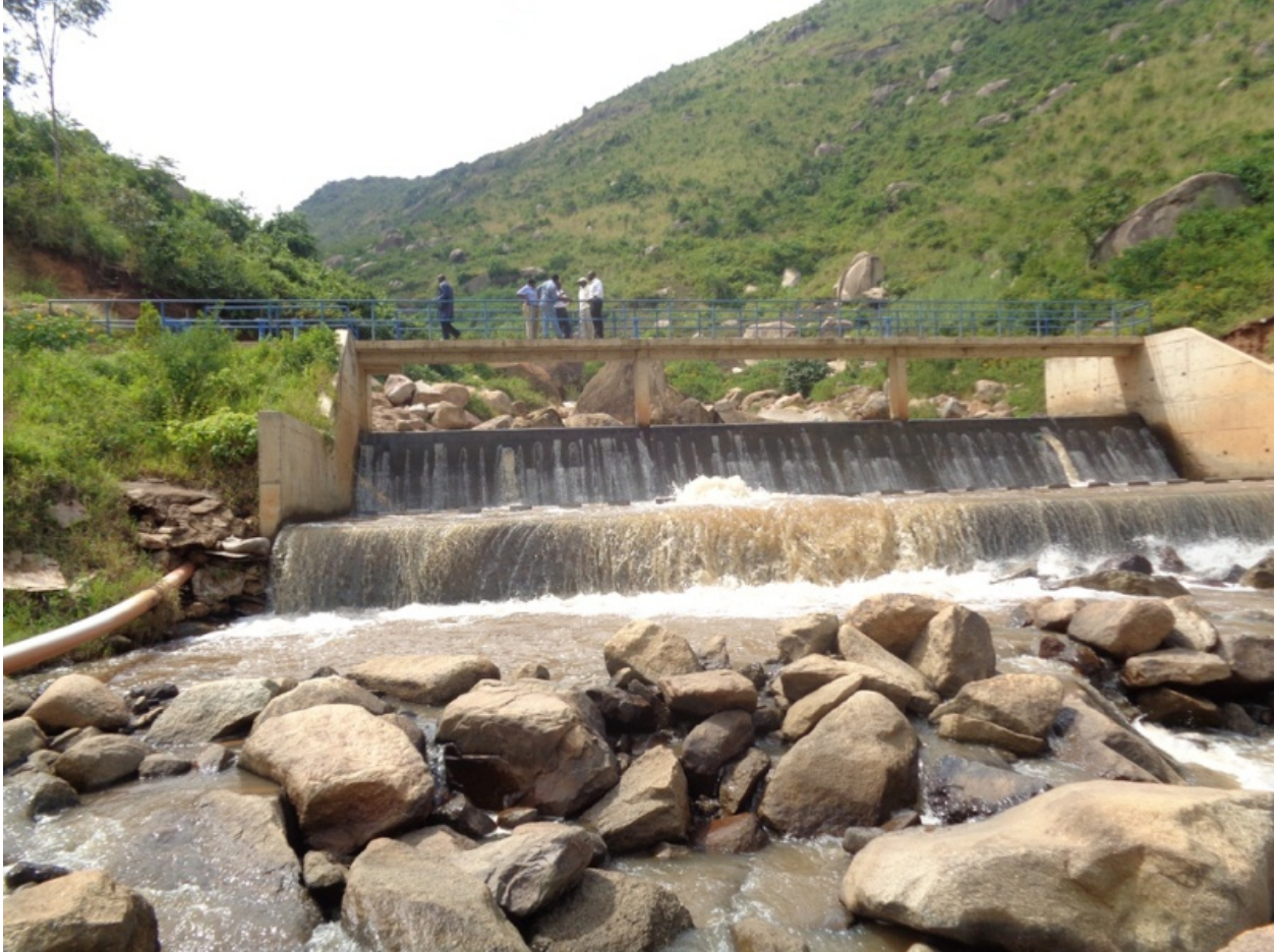
Plate 7: Kajulu water intake. This intake supplement water from the Dunga water works on the shores of Lake Victoria. The intake suffers high turbidity during rains and low volumes and high contents of cations during dry seasons.
